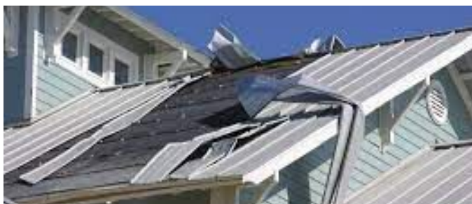
METAL PANEL DAMAGE
