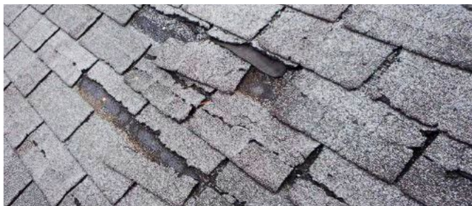
SHINGLE CRACKING & CURLING
