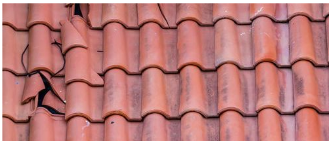
MISSING AND CRACKED TILE
